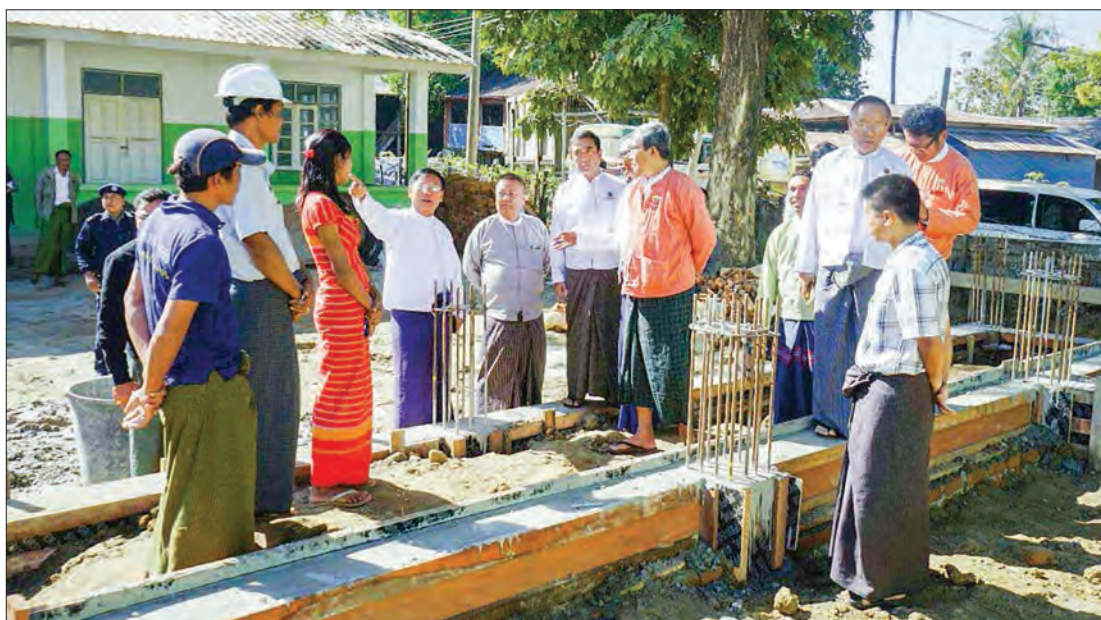
Rakhine State Chief Minister U Nyi Pu and departmental officials inspect the construction of a new school building in Yanbye Township. PHOTO: MNA
