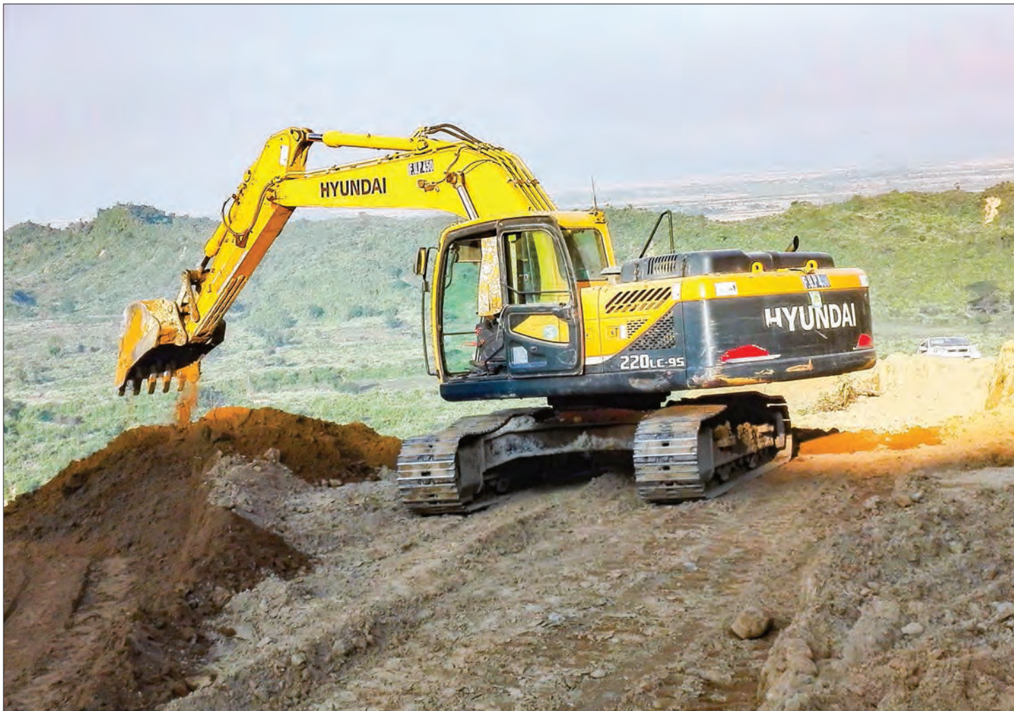
The backhoe working on the road construction in Maungtaw, Rakhine State. PHOTO: NAY WIN TUN
