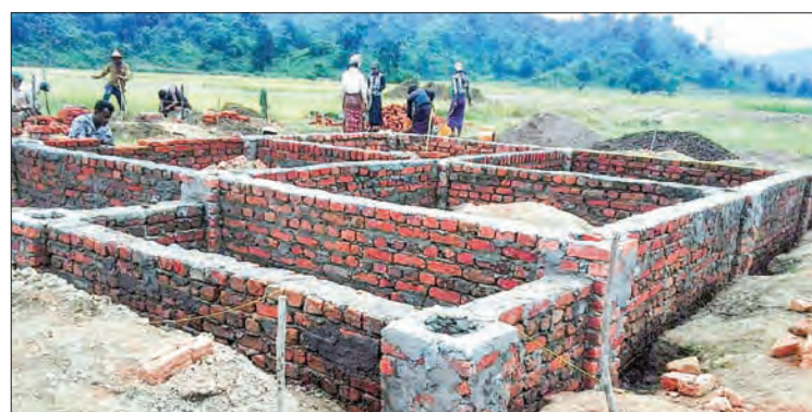
Workers constructing houses for four villages of ethnic Mro villagers in Maungtaw District. PHOTO: MIN HTET
