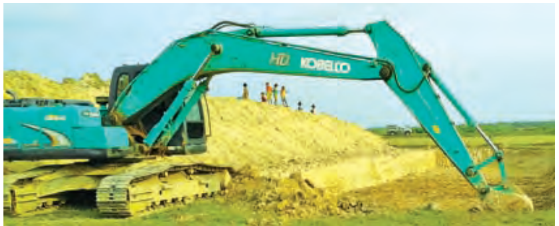
A fish pond is being dug with the use of heavy machinery in Maungtaw. PHOTO: MAUNG MAUNG THANT
