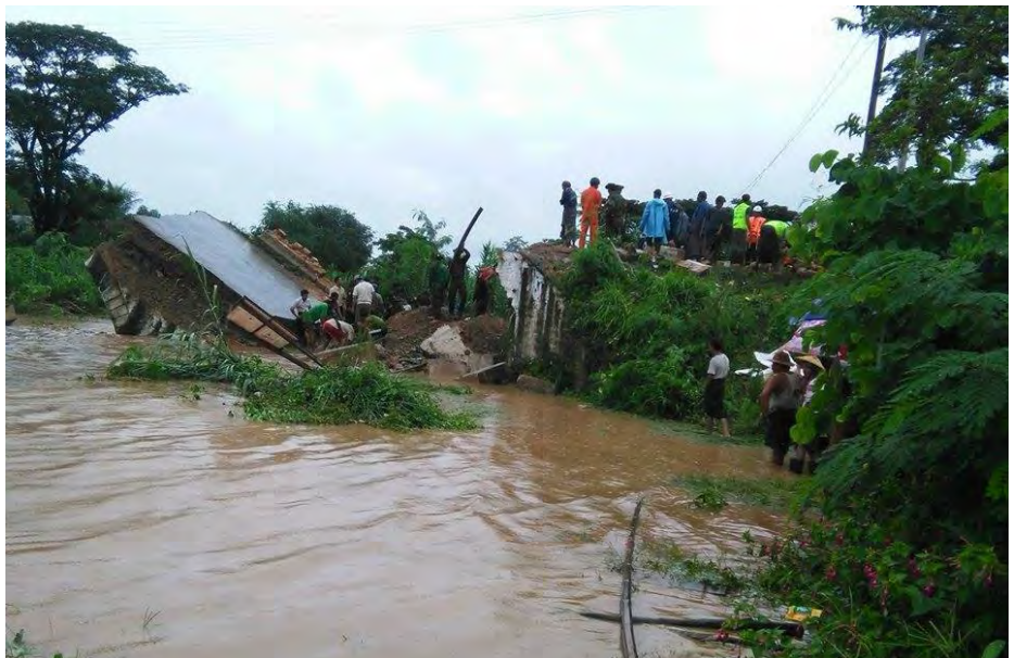
Damage caused by flooding in Hsipaw in July 2015
