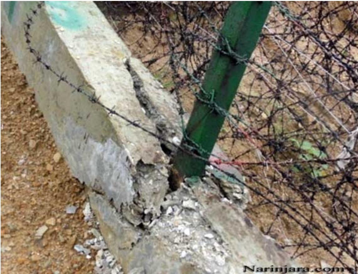
Border fence destroyed at the Bangladeshi side
