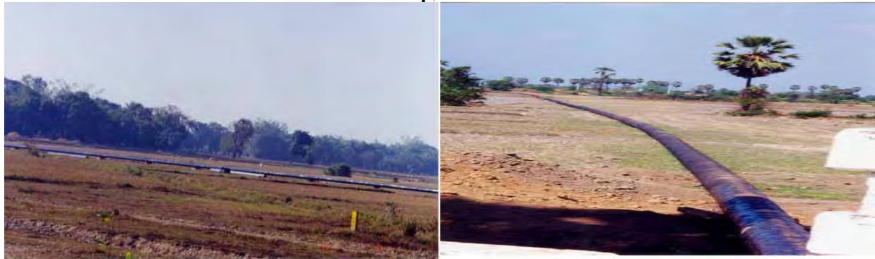
Gas pipeline crossing on private farm, Nyaungbinseik & Kyawechangone village, Kyeikmaraw Township, Mon State
