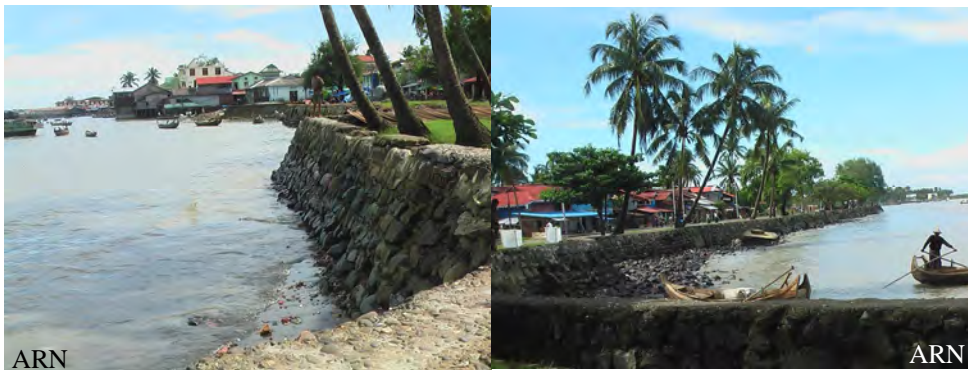
Proposed Port area of Kaladan Multi-Modal Transit Transport Project along the Strand Road of Site-tway
