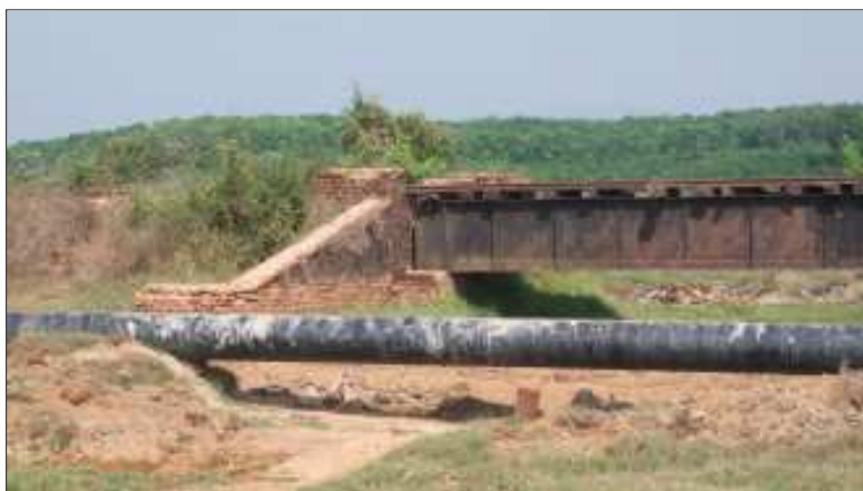
A exposed portion of the old Kanbuak to Myaing Kalay pipeline is seen as it crosses over a dry creek bed near Lamine sub-township
