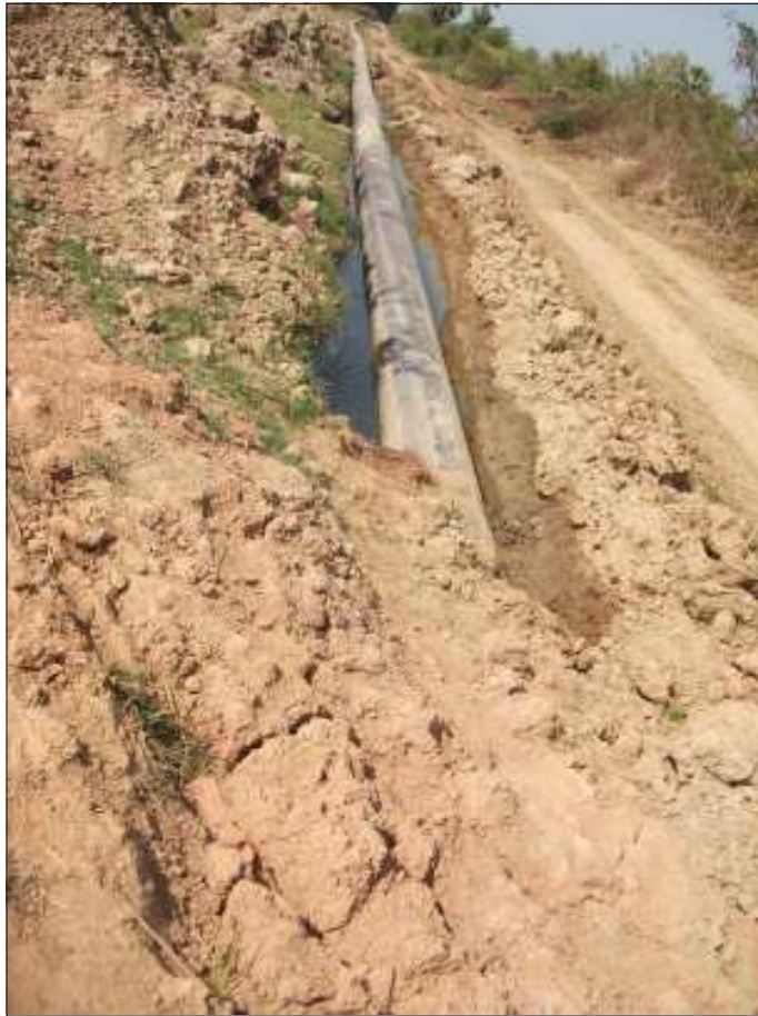
A portion of newly laid pipeline is seen recently installed, waiting to be recovered by village laborers from Lamine sub-township.
