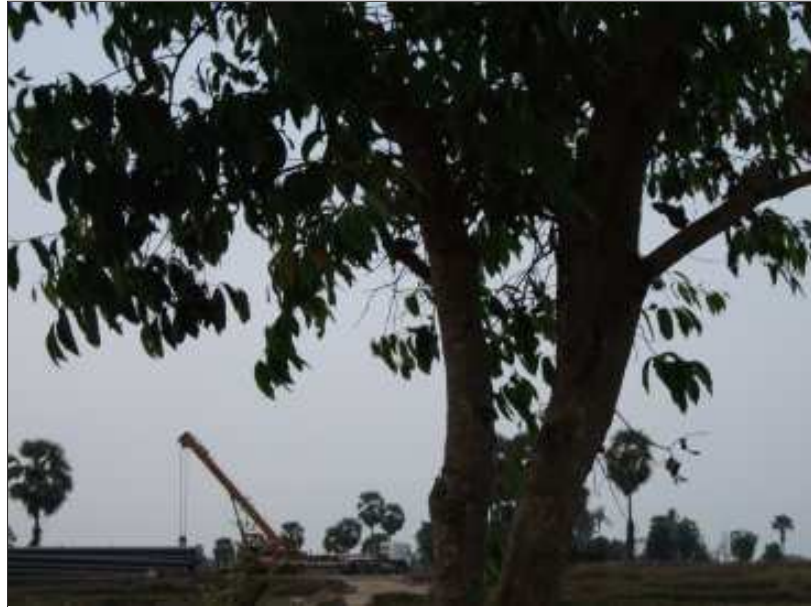
A crane belonging to MOGE is seen installing new pipes on the Kanbawk to Myaing Kalay near Lamine sub-township.
