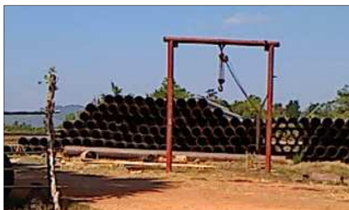
A stack of pipe segments is seen a transfer station where segments will be sent to portions of the pipeline that will be completed.
