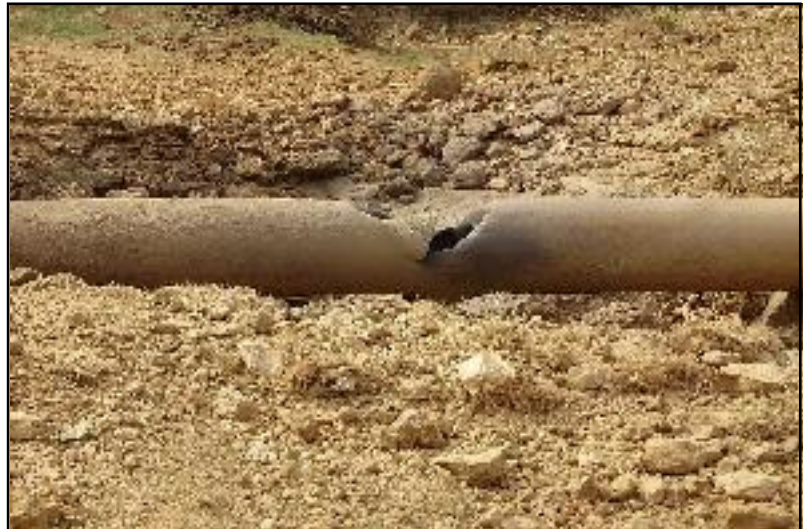
A portion of the Kanbawk to Myaing Kalay natural gas pipeline is seen exposed after a rupture near Lamine Sub-township, Ye Township, Mon State
