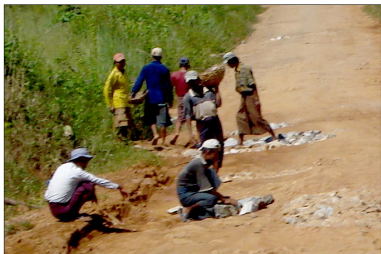
Villages are forced to perform road repairs near Yapu village in November 2008.
